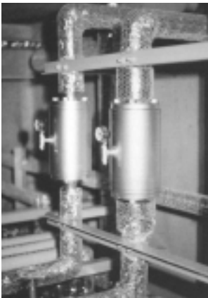
Installation in riser for lift pump
