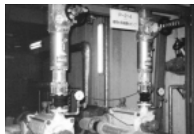
Installation in riser
